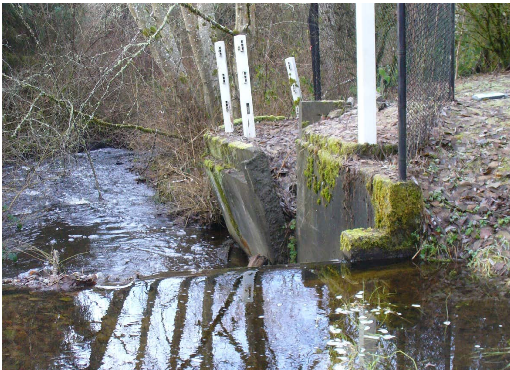
Figure 16. Facing downstream (south) from just above the weir. Note failing concrete wall which was a former footbridge abutment (12/15/22).
