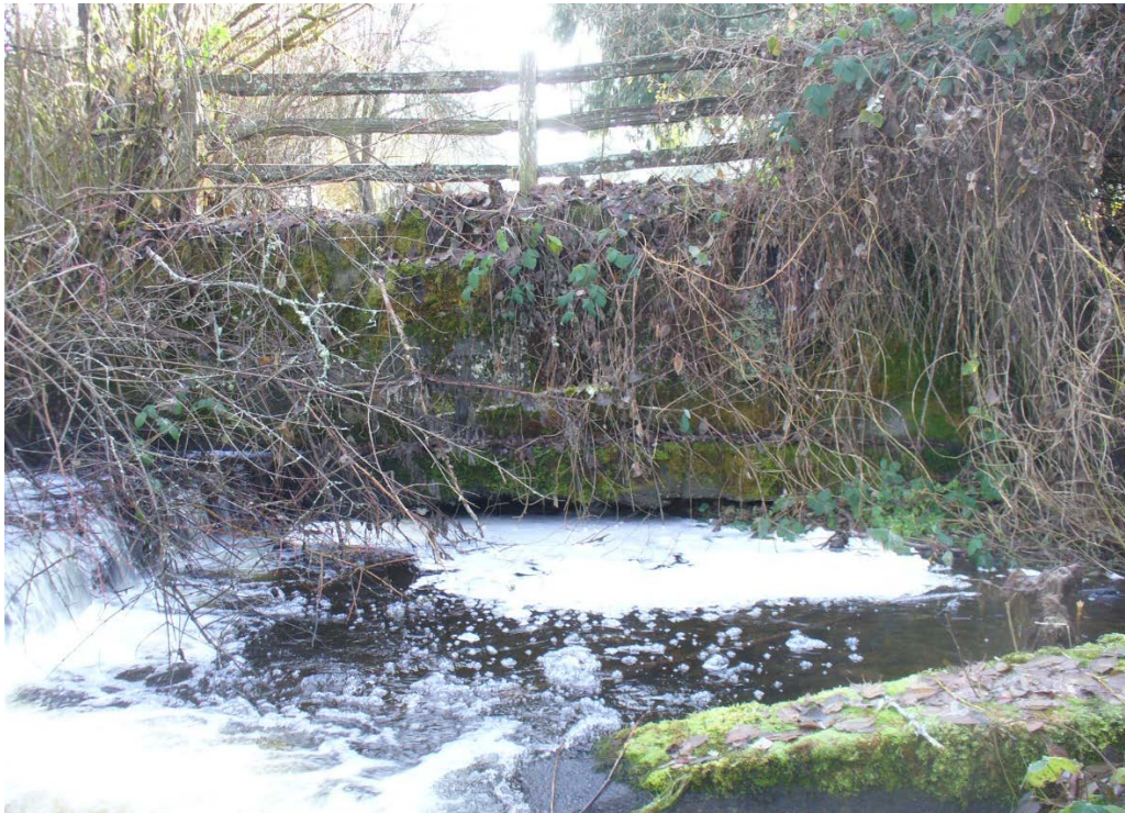
Figure 18. Facing east, vertical streambank just below the weir, beyond which is the Homestead community (12/15/22). Note undercut, failing support wall.
