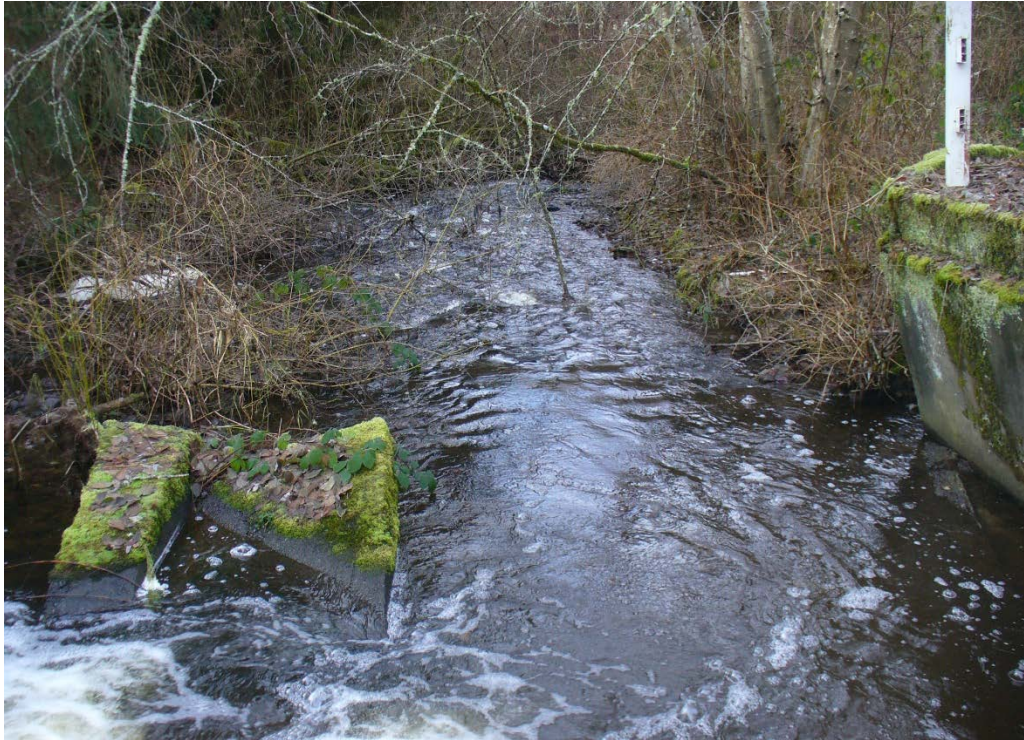
Figure 17. A view of the channel facing south, downstream. The concrete in the channel on the left side is a toppled center support for the former footbridge (12/15/22).
