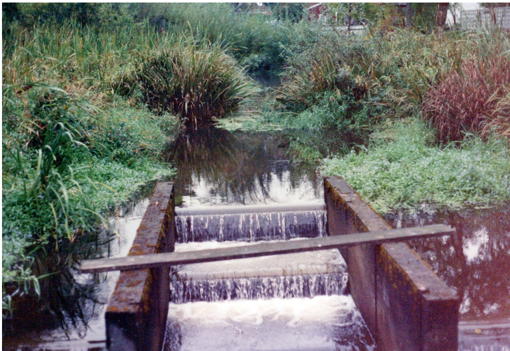
Figure 20. Fish ladder and area upstream in October of 1990 showing backwatered condition and emergent vegetation.
